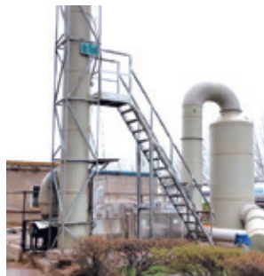
Waste Gas Treatment Equipment of the Sewage Tank—Dispose of Foul Smell of Sewage 污水池的廢氣處理設備 — 處理污水臭味
