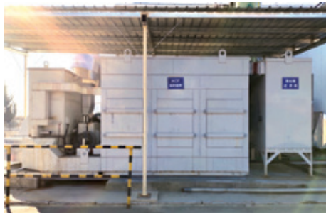
Organic Waste Gas Catalytic Combustion Purification Device 有機廢氣催化燃燒淨化裝置
