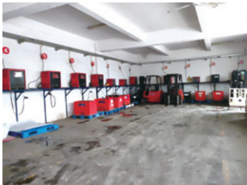
Forklift Charging Room 叉車充電間
